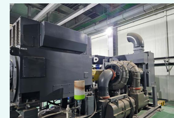
Pohang Cathode Materials Plant compressor
