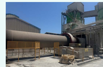
Refractory Rotary Slaker
